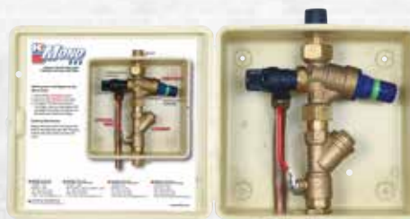
House Water Station
