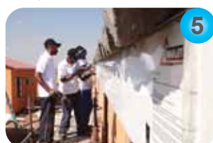
Fix Fascia Fix far side of fascia with non-corrosive screws for steel trusses and nails for wood trusses.
