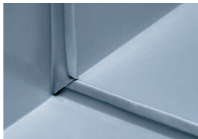
Pinched seam on roof penetration (2) Apron area
