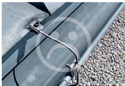
Lightning protection Fix panel on point of eave = expansion cracks on panel
