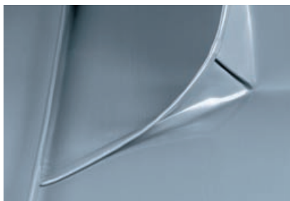
Rounded seam connection (1a) Upstand ≥ 150 mm with water check, pinched seam round seamed to double standing seam
