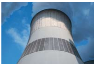
Chimneys and cooling towers
