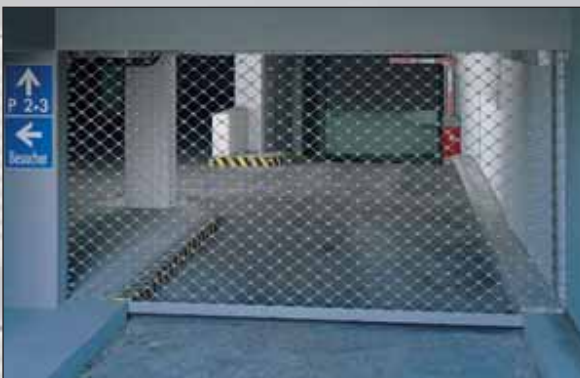
Security and ventilation in underground garages.
