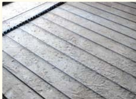
Underfloor heating should be installed at this point
