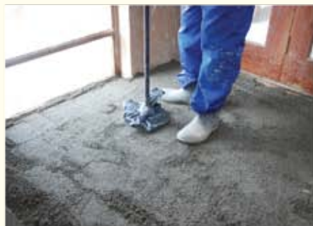
Place the screed to a minimum thickness of 30mm and compact thoroughly. The placing of the screed should take place while the slurry coat is wet
