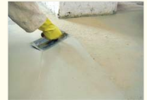
Steel float immediately to a very smooth finish. Leave the completed floor to dry for 24 hours
