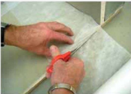
Cut membrane to size, allowing the joints to overlap by 100mm with neighbouring membrane.
